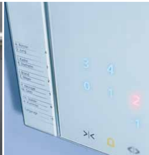
Nameplate for Glass Car Operating Panel
